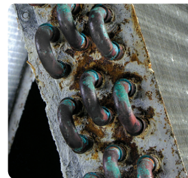
Copper tube and galvanized tube sheet after 500 hour salt spray.
