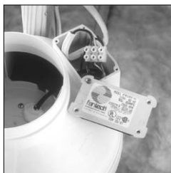
Romex wiring – Top View
