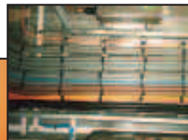
Marine Cable Bundling
