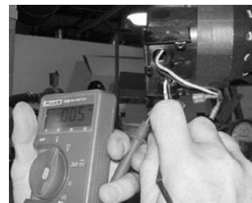
Checking line voltage at the blower wire harness connection on blower.
