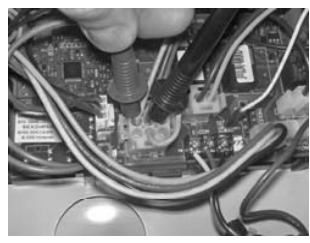
Checking MV pin terminal to gas valve wire harness for 24 volts output to gas valve during heating cycle (pilot must be lit with no sparking).
