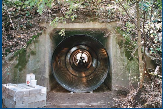
Corrugated Steel Pipe was used to repair a failing reinforced concrete box under a height of cover of 91 feet. Grout plugs were furnished to facilitate concrete grout placement between the new corrugated steel pipe and the existing concrete box.
