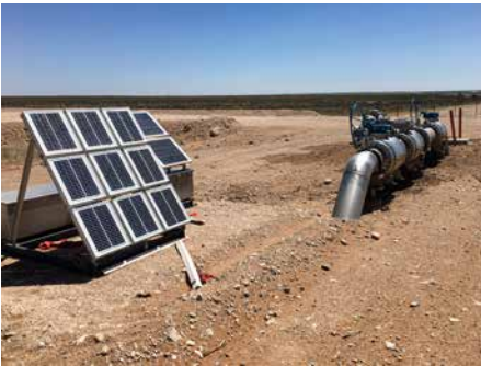
Figure 4: A rigorous evaluation of the solar-powered valve packages validated the expected performance signatures.
