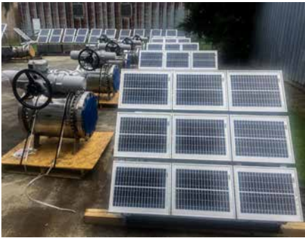
Figure 2: Pipeline control stations employ 12 and 16-inch ball valves automated with electric actuators. Each valve has its own solar panel.
