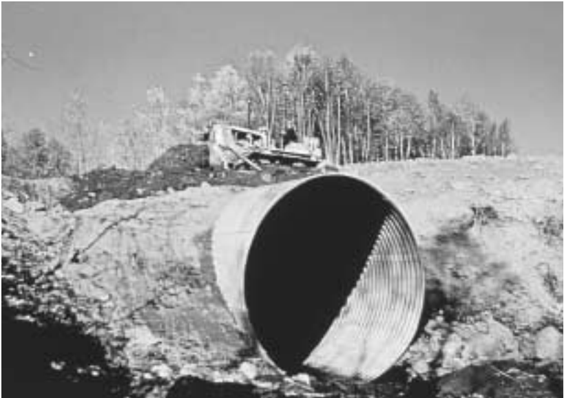
Figure 19. Compacted side fill should be completed on both sides of structure before fill is "carried over" for construction traffic.
