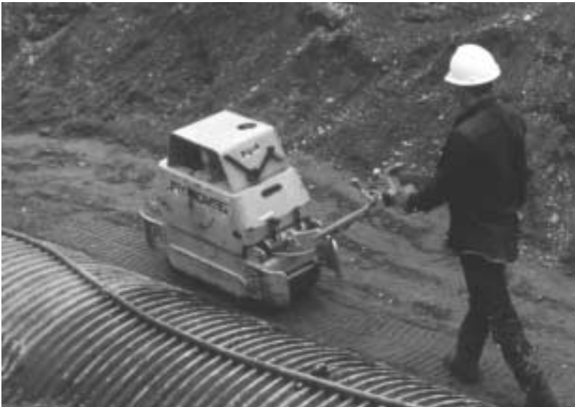
Adequate, uniform compaction is the secret to building soil and steel structures.
