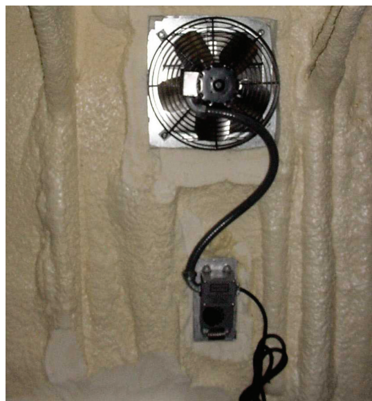
Complete Exhaust Fan (Interior View)
