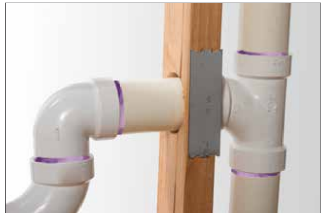
Stud Protection Needed. Drain line in second stud bay needs added protection and reinforcement.
