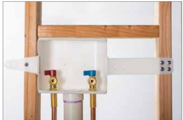
Inferior Bracketing. Contractors are forced to add their own wood braces to supplement flimsy styrene brackets.
