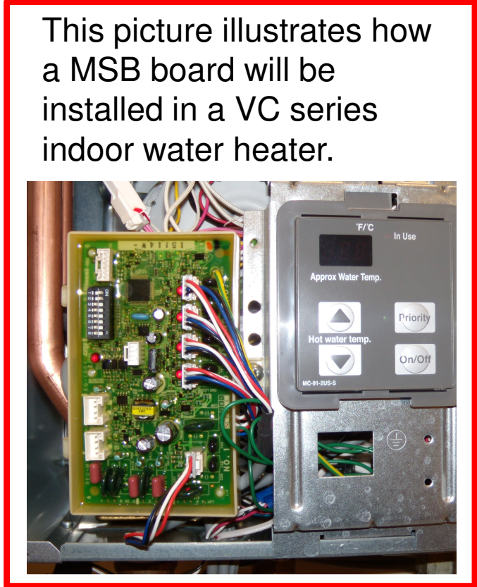
Cables linking the MSB to other water heaters.
