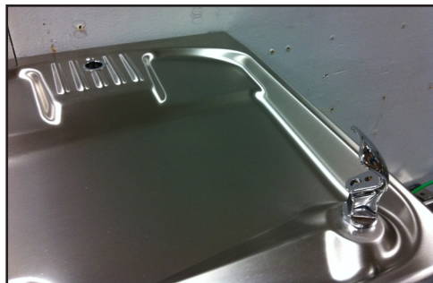
Exchange Bubbler hardware.
