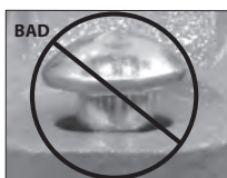
OVAL NECK OF BOLT NOT SEATED PROPERLY
