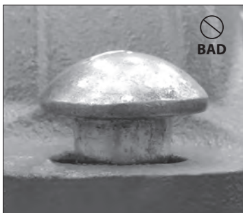
BAD BOLT ENGAGEMENT (OVAL NECK IS NOT SEATED PROPERLY IN THE BOLT HOLE)
