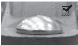
GOOD BOLT ENGAGEMENT (OVAL NECK OF EACH BOLT IS SEATED PROPERLY IN THE BOLT HOLE)
