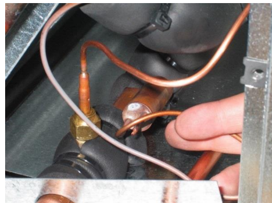
Figure 27. Thermal Measuring Bulb Placed on Copper Tube.
