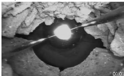
Figure 13 – Typical Crossbore Into Sewer Line
