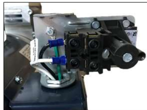
6. Insert spade connector into other motor terminal. Use wiring diagram on side of motor to wire it for 230V. 7. Wire supply line 1 and line 2 to line contacts of pressure switch.
