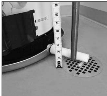
Figure 26 - Temperature and Pressure Relief Valve Pipe
