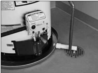
Figure 23 - Metal drain pan piped to drain.
