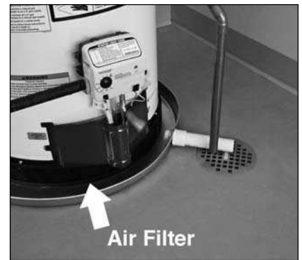
Figure 24 - Filter attached to water heater.
