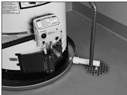
Figure 23 - Metal drain pan piped to drain.
