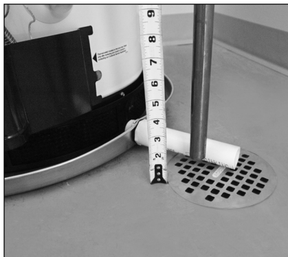
Figure 26 - Temperature and Pressure Relief Valve Pipe
