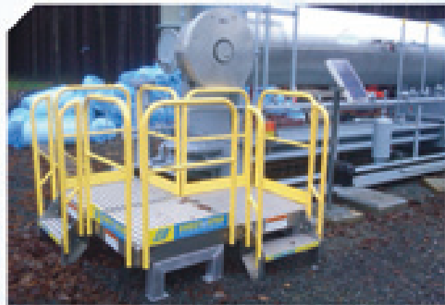
Platform allowing access to two sides of pumps.
