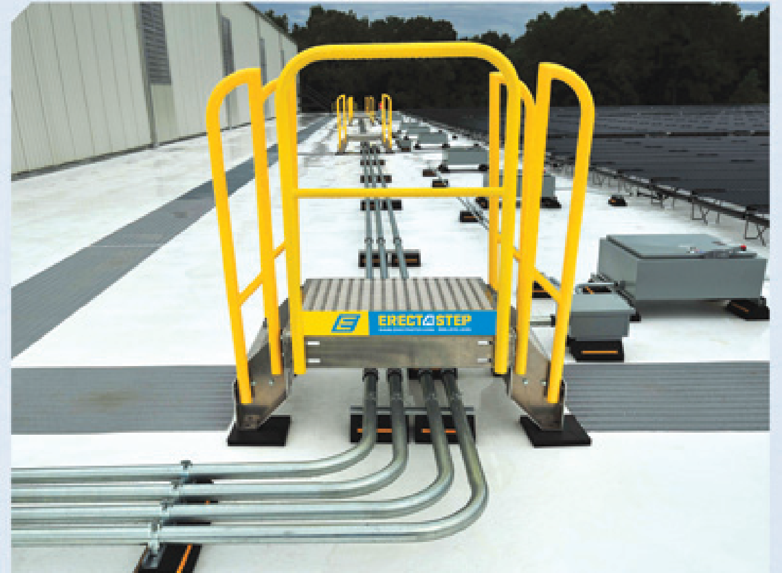
Rooftop access to solar and air conditioning units.
