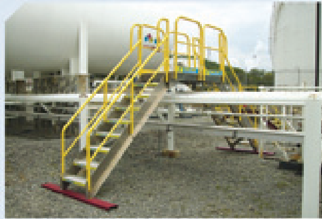
Eight stair pipe crossover.
