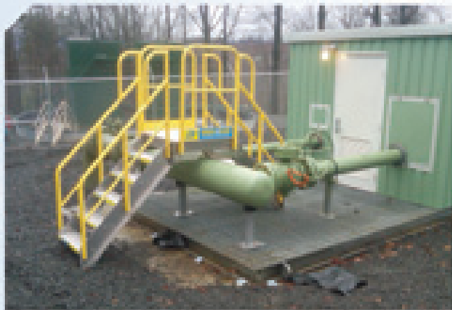
Pump station access was an afterthought.
