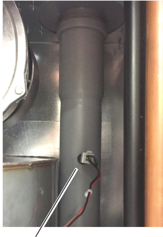
Flue temperature and flue safety sensors
