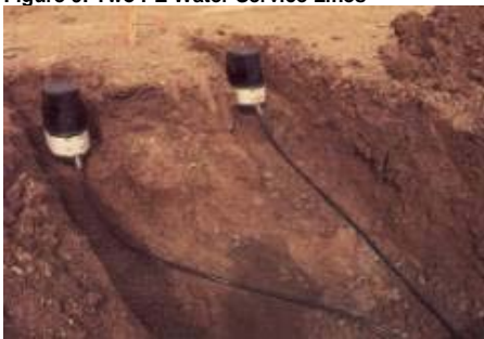
Figure 9: Two PE Water Service Lines
