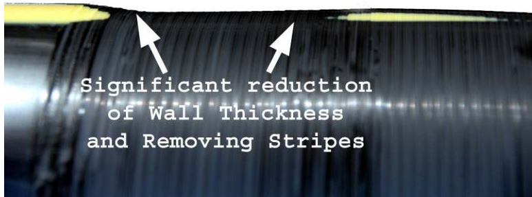
Figure 69: Over Scrape Unacceptable – Possible Causes: Incorrect Scraper, Poorly Maintained Scraper, Excessive Number of Passes with Scraper and Ineffective Evaluation of Scraping
