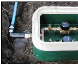
19a: Meter Box Mechanical Coupling
