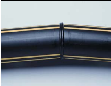
Figure 42: Visually unacceptable mitered joint
