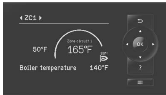
Display - Zone circuit operation
