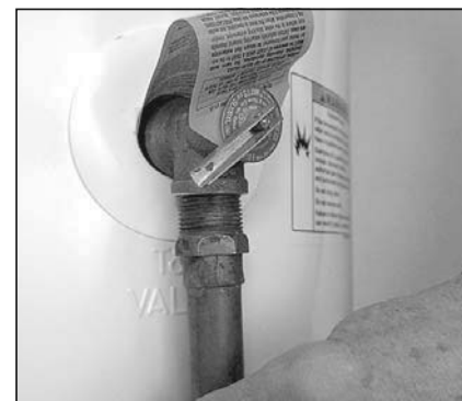
Figure 16 - The T&P Relief Valve discharge pipe must be installed properly and piped to an adequate drain.
