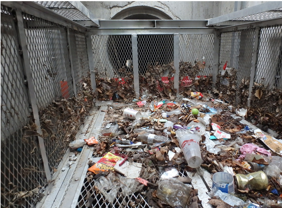
Nutrient Separating Baffle Box with collected trash, organics and debris inside the screened basket system ready for disposal.
