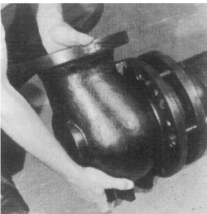
3. Slip off Hydrant Shoe.
