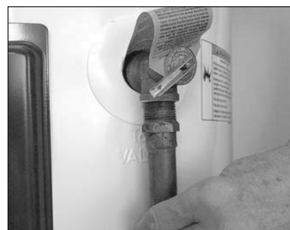
Figure 16 - The T&P Relief Valve discharge pipe must be installed properly and piped to an adequate drain.
