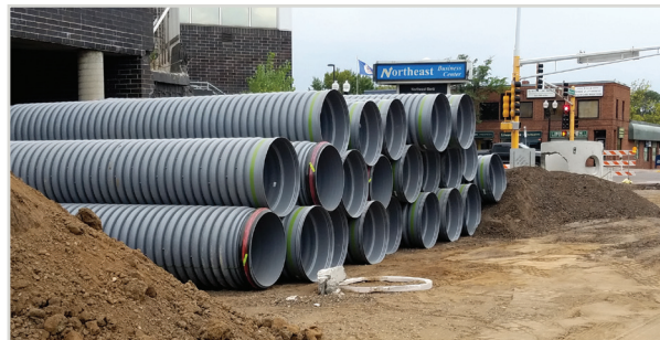
While supporting lengths of pipe evenly, alternate bells for each row of pipe.
