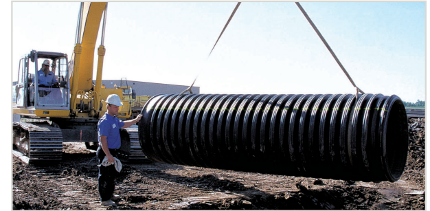
Lift 36"-60" (900-1500 mm) diameter pipe with a sling at two points, spaced 10' (3 m) apart.
