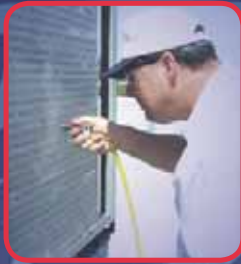
Blow off coils with Sludge Sucker® Blowgun
