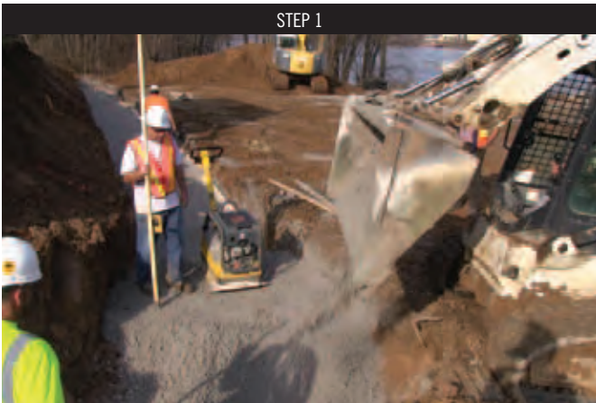
Place the 6" crushed stone ( 3/4" rock) to create the leveling pad for the Mega-Tandem™ (MSRW).
