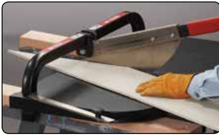
Scribe desired angle on fiber cement siding plank and feed it into the guillotine blade as you cut.
