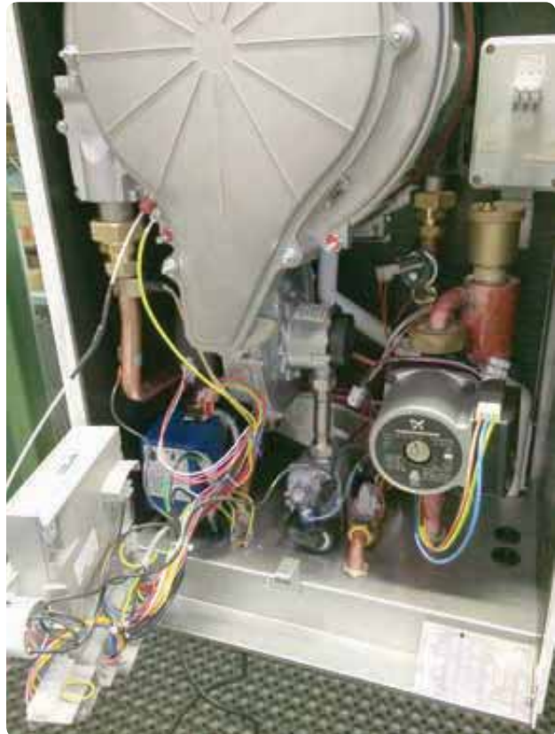
Figure 140 Boiler front panel removed
