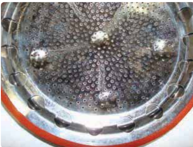
Figure 143 Inspecting interior and cleaning the burner
