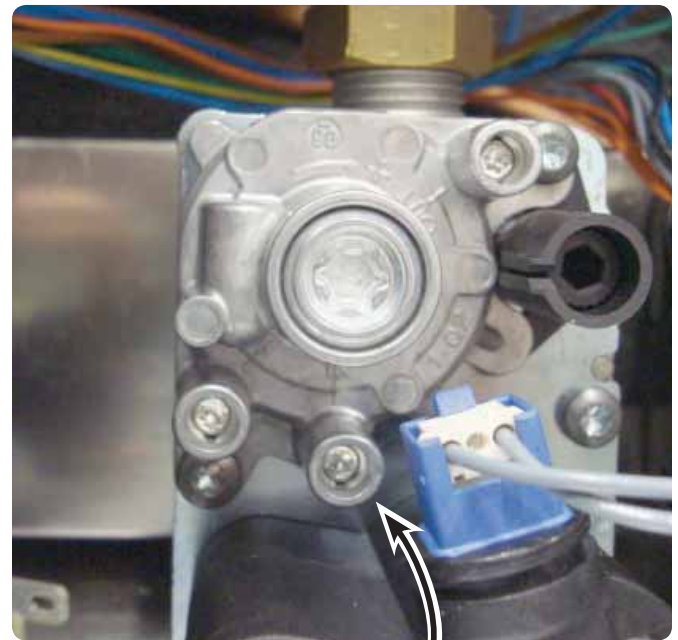
Figure 64 Inlet test port on gas valve
