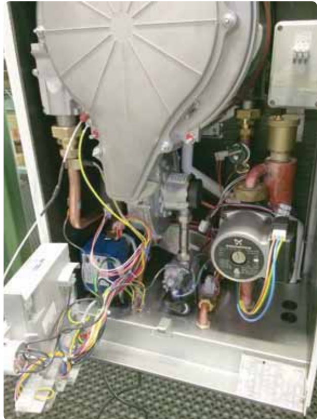
Figure 144 Boiler front panel removed
