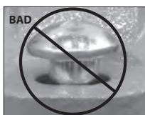
OVAL NECK OF BOLT NOT SEATED PROPERLY
