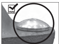
OVAL NECK OF BOLT SEATED PROPERLY
