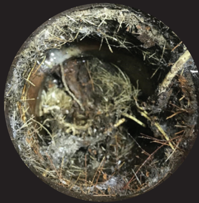
SEMI-HARD BLOCKAGES Light Tree Roots, Plant Roots
