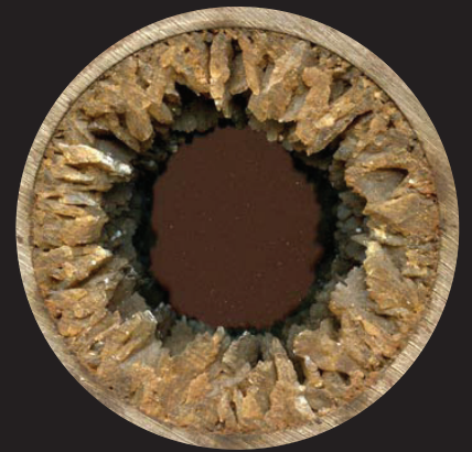
HARD BLOCKAGES Scale, Uric Scale, Limestone
