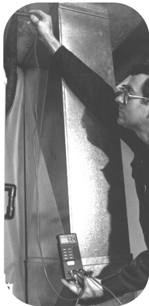
FIGURE 48 TEMPERATURE RISE MEASUREMENT
