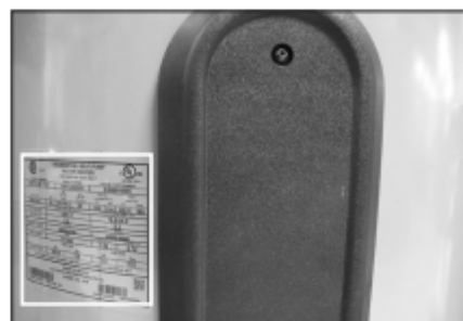
Figure 22 - The water heater's electrical requirements can be determined from the data plate.
