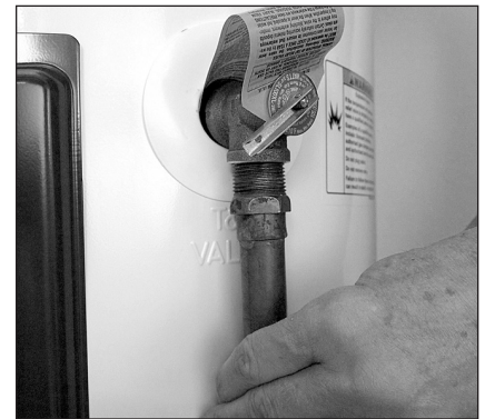
Figure 15 - The T&P Relief Valve discharge pipe must be installed properly and piped to an adequate drain.
