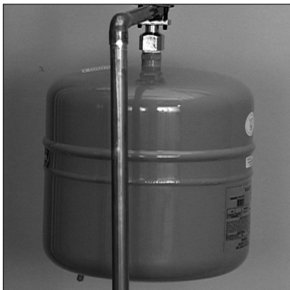
Figure 19 - The Thermal Expansion Tank should be pressurized with air to match the home's incoming water pressure.
